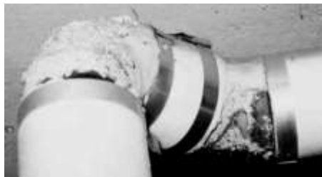
Damaged Pipe Insulation
